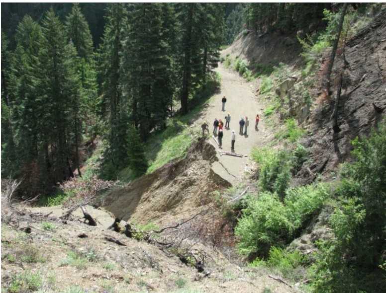
Photo 13 (#2981) - Road Fill Failure Hawkins Creek Watershed 5-17-13 Jdlf
