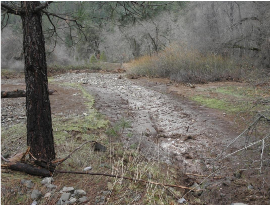
Photo 16 - Wheeler Ranch Road Wash-out 12-14-2012
