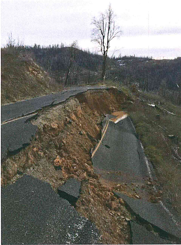
Storm damaged road in the Cornerstone area of the Stanislaus National Forest.
