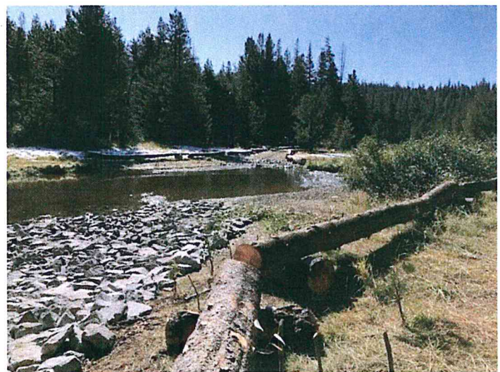
Defined and delineated the crossing at Deer Creek using local materials to reduce the occurrence of user created routes and their effects on riparian vegetation. Photo by US Forest Service
